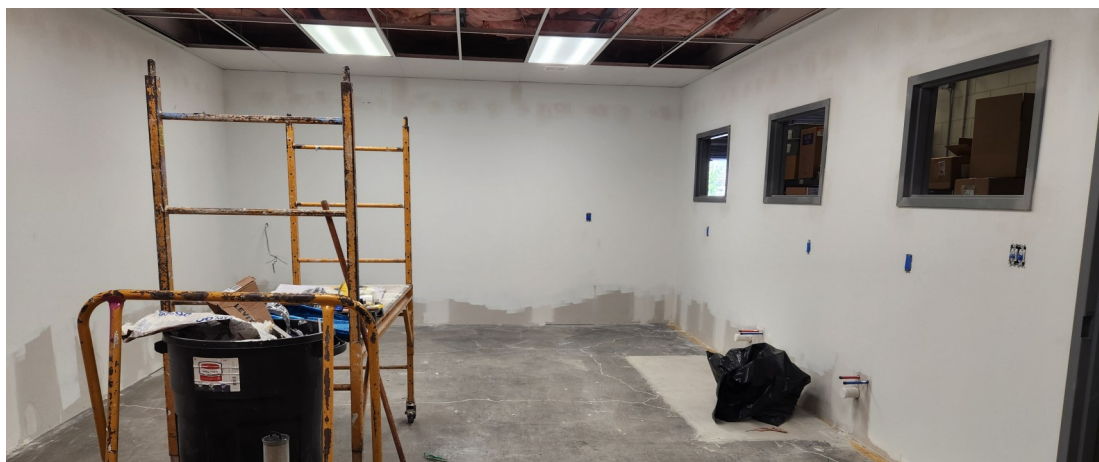
The construction phase of the upgraded quality testing laboratory in R&R's Maumee, OH production facility
